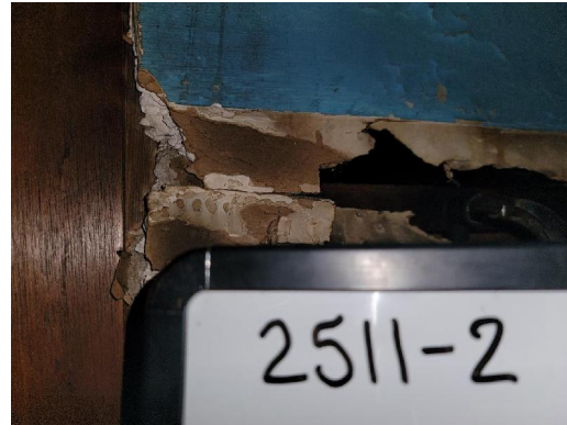
2511-2 Drywall Joint Compound (2% Chrysotile) Typical Interior Walls
